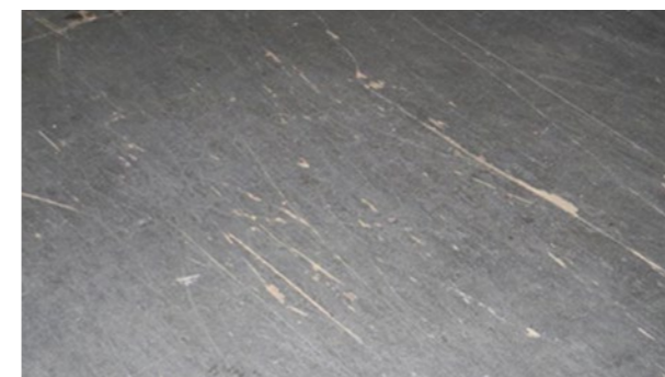
☰ Flooring: Slight deformation, superficial wear
